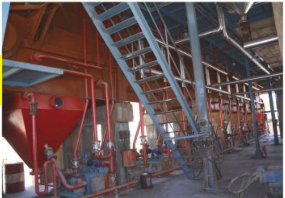
View of Pump Section Solvent Extraction Plant
