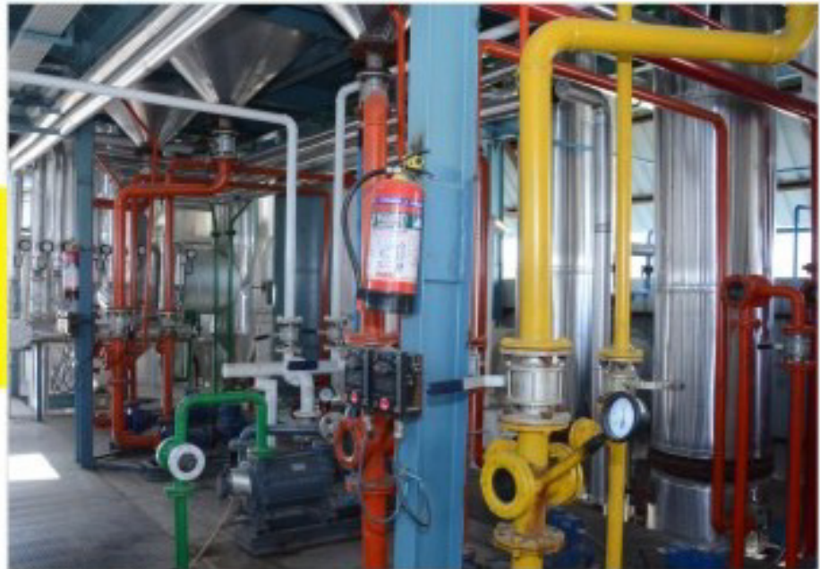
Internal View Solvent Extraction Plant
