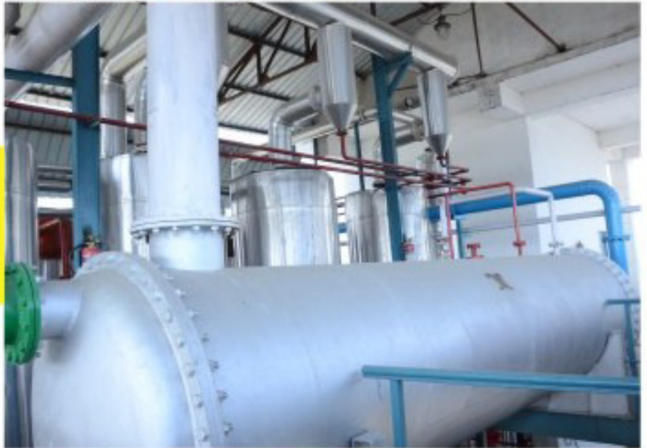
Internal View Solvent Extraction Plant
