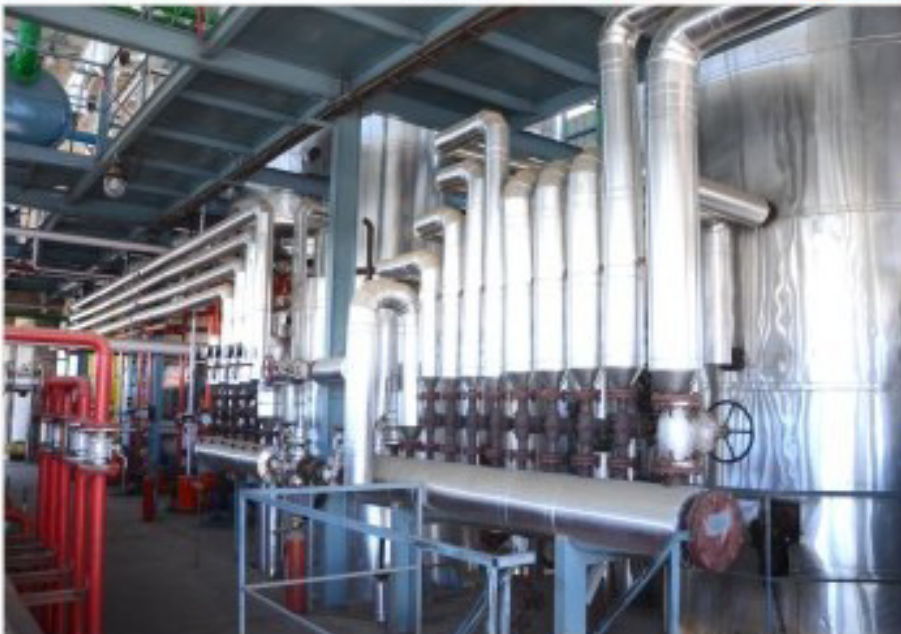
Internal View Solvent Extraction Plant
