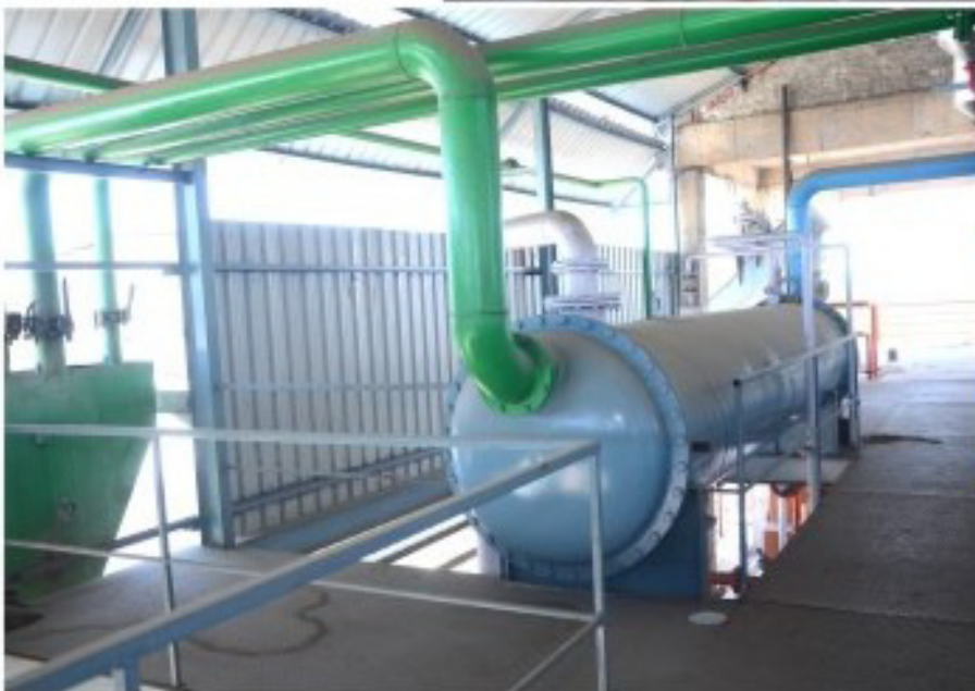
View of Water Header Solvent Extraction Plant
