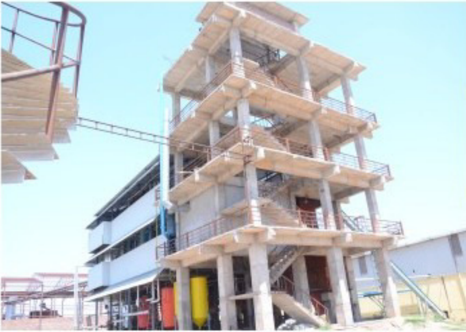
Solvent Extraction Plant Capacity 800 TPD,
